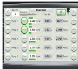
Operating The dosage and the mix of chemicals is controlled from the drivers cabin.
